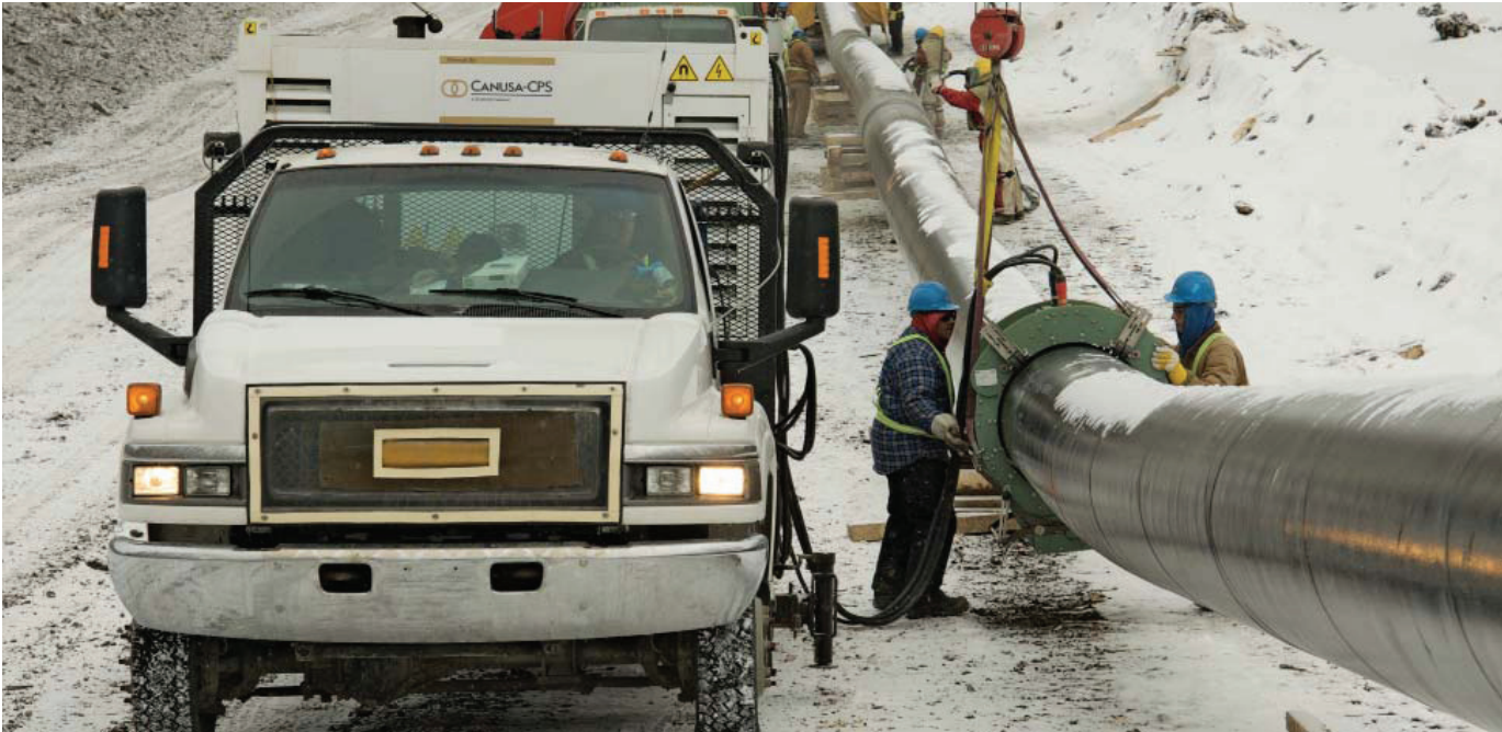
Every season is the right season for pipeline safety. Applying heat-shrinkable sleeves on pipelines sometimes requires technicians to work in all manner of climates to ensure pipelines are protected from corrosion.
