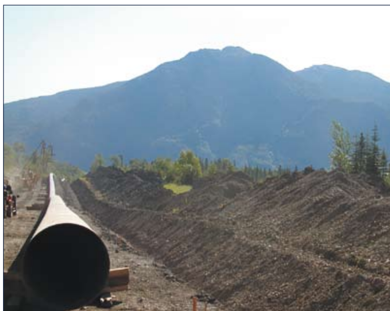
Figure 5. Aggressive construction conditions.
